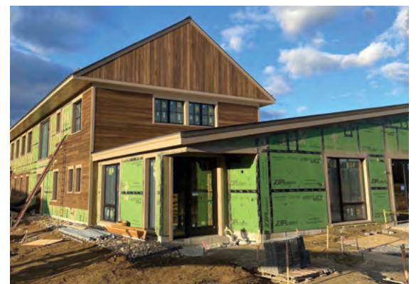
The Mathey Center close to its final form. COURTESY OF CHAPMAN DESIGN/CONSTRUCTION
